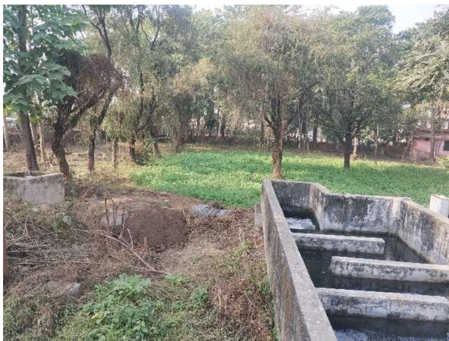
Picture 4-2: Irrigation canal of Jagjeetpur STP
